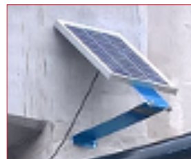
Solar panel for 3G gateway
